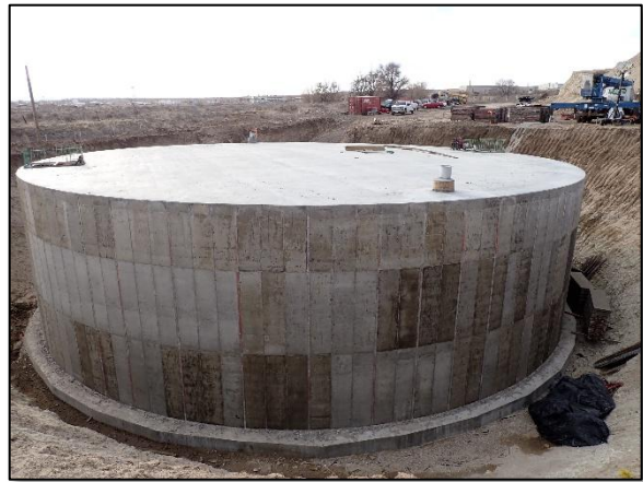
Image 5.) Zone 3, 0.75 MG Underground Tank
