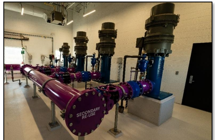
Image 4.) MWD's WRF Reuse Supply Pumps
